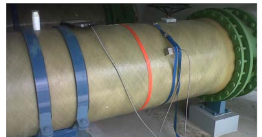
KATflow 230 and K0 transducers installed on large fiberglass pipe
